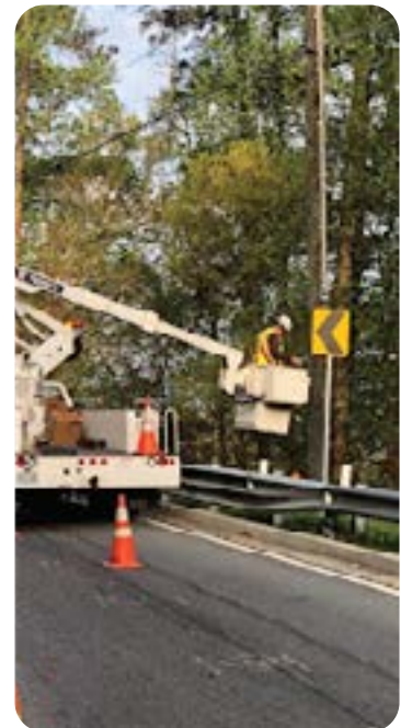
City Foot Traffic Street Electric & existing pole
