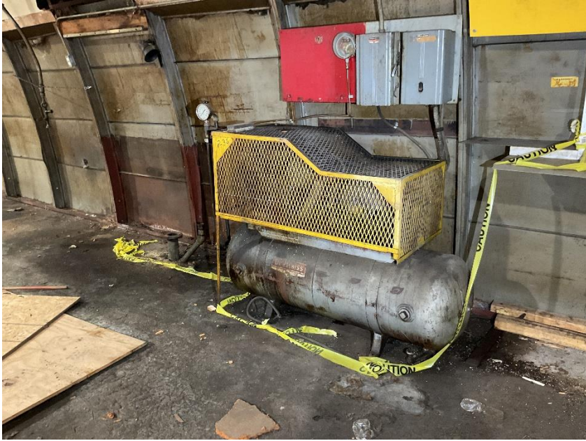
Air compressor located in the central shop area
