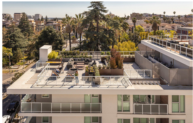
Roof-mounted mechanical equipment concealed behind screens.
